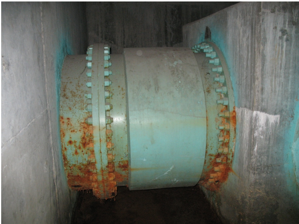
Figure 6 - Existing 1200 mm Pipe Spool to Pump Station - To Be Repaired
