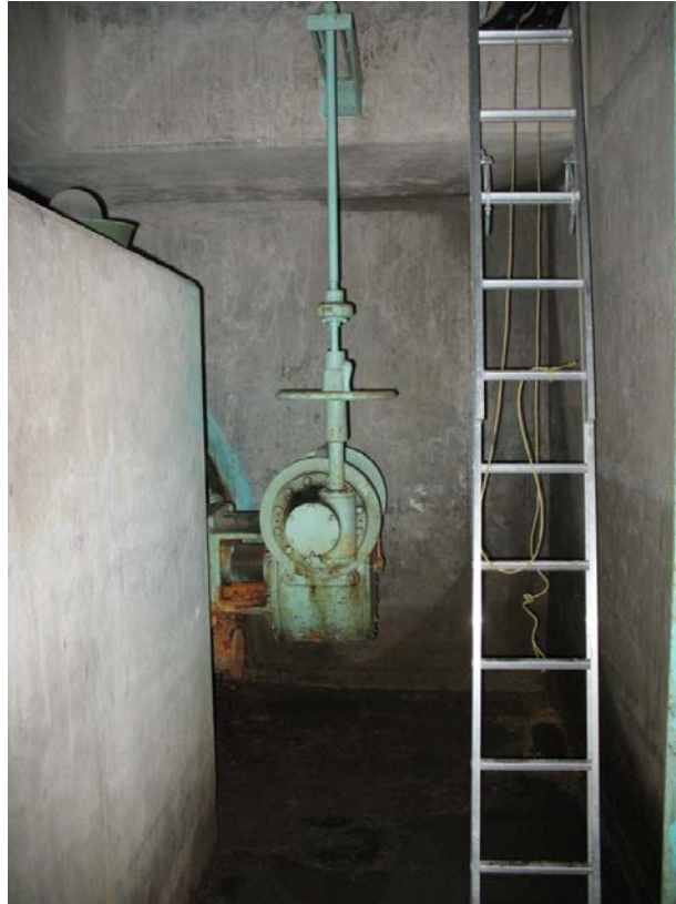
Figure 5 - Existing 1200 mm Valve Actuator
