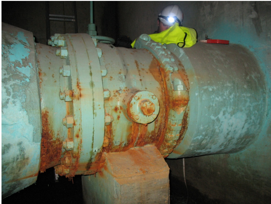
Figure 7 - Existing 900 mm valve, Reducer and Spool Pipes - To Be Repainted
