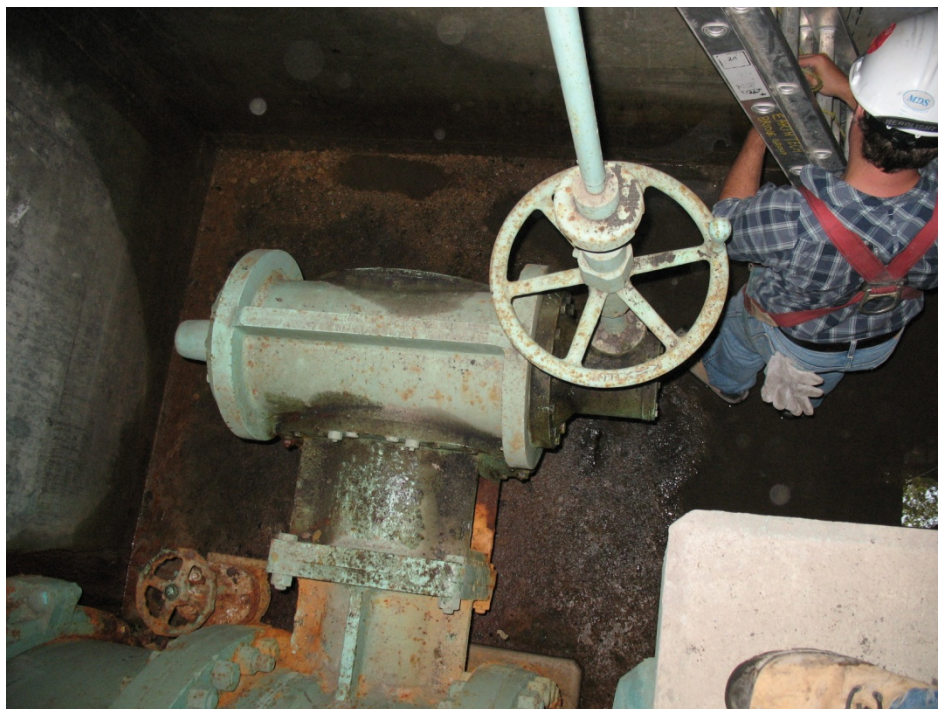
Figure 2 - Existing 1200 mm Valve Actuator
