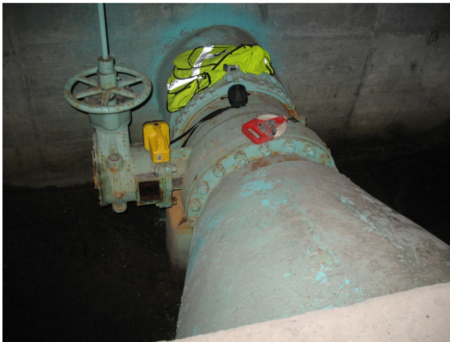
Figure 8 - Existing 900 mm valve, Reducer and Spool Pipes - To Be Repainted
